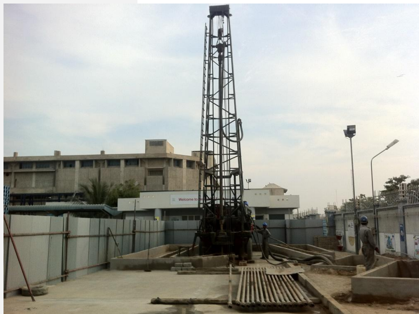
1500 ft water well for Nestle on behalf of Schlumberger Water Services, Abu Dhabi.
